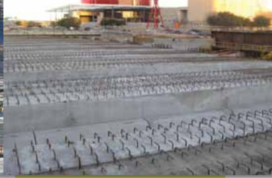
LEFT: Arrival of beam for signing ceremony. CENTER: Cranes lift beams into place. RIGHT: The beams create the foundation for The Park
